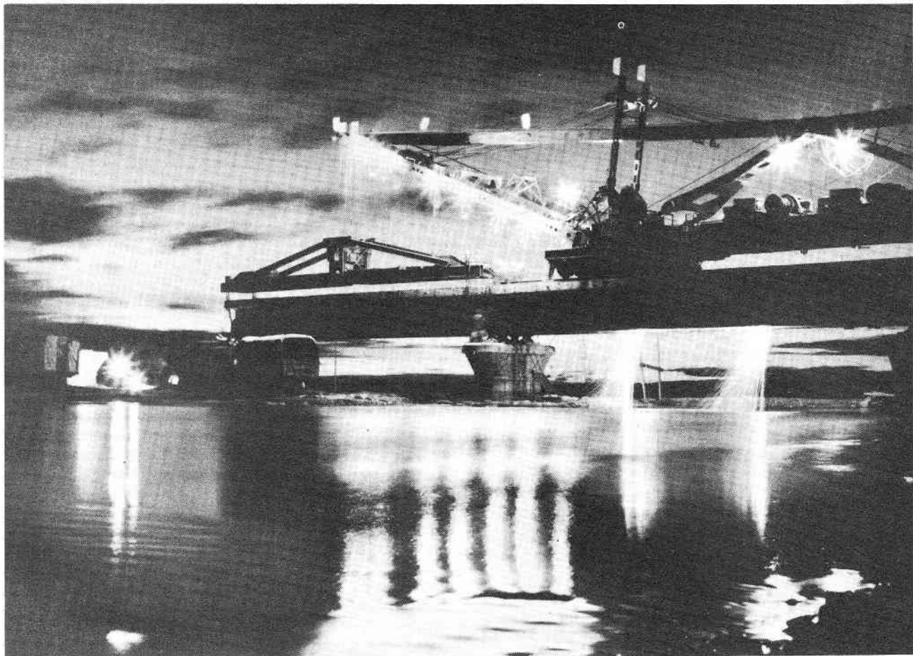
A bridge over the Buha River on the Qinghai-Tibet line being built by the P.L.A. railway corps.
