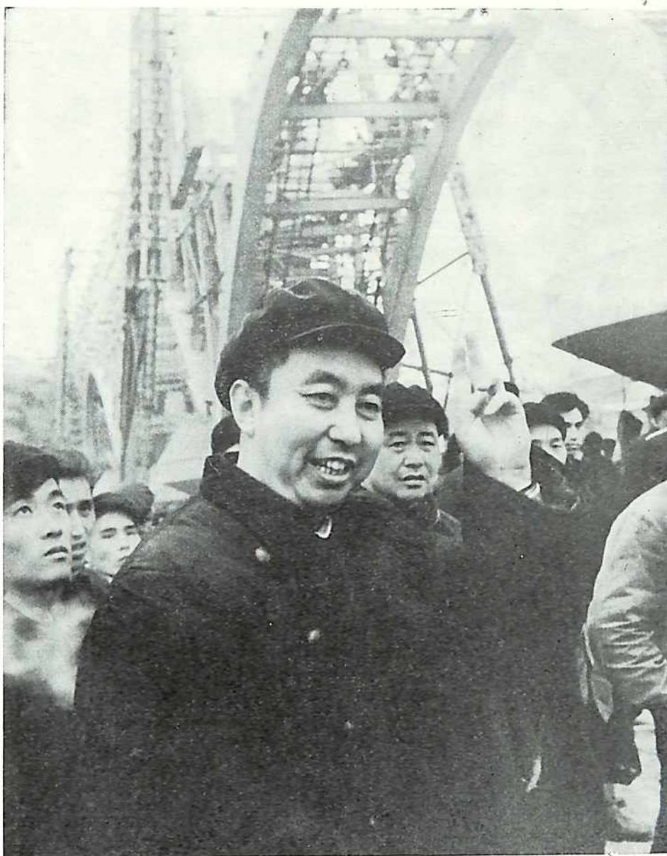
Comrade Hua Kuo-feng at the Chuchintu worksite of the Shaoshan irrigation project, January 1966.
