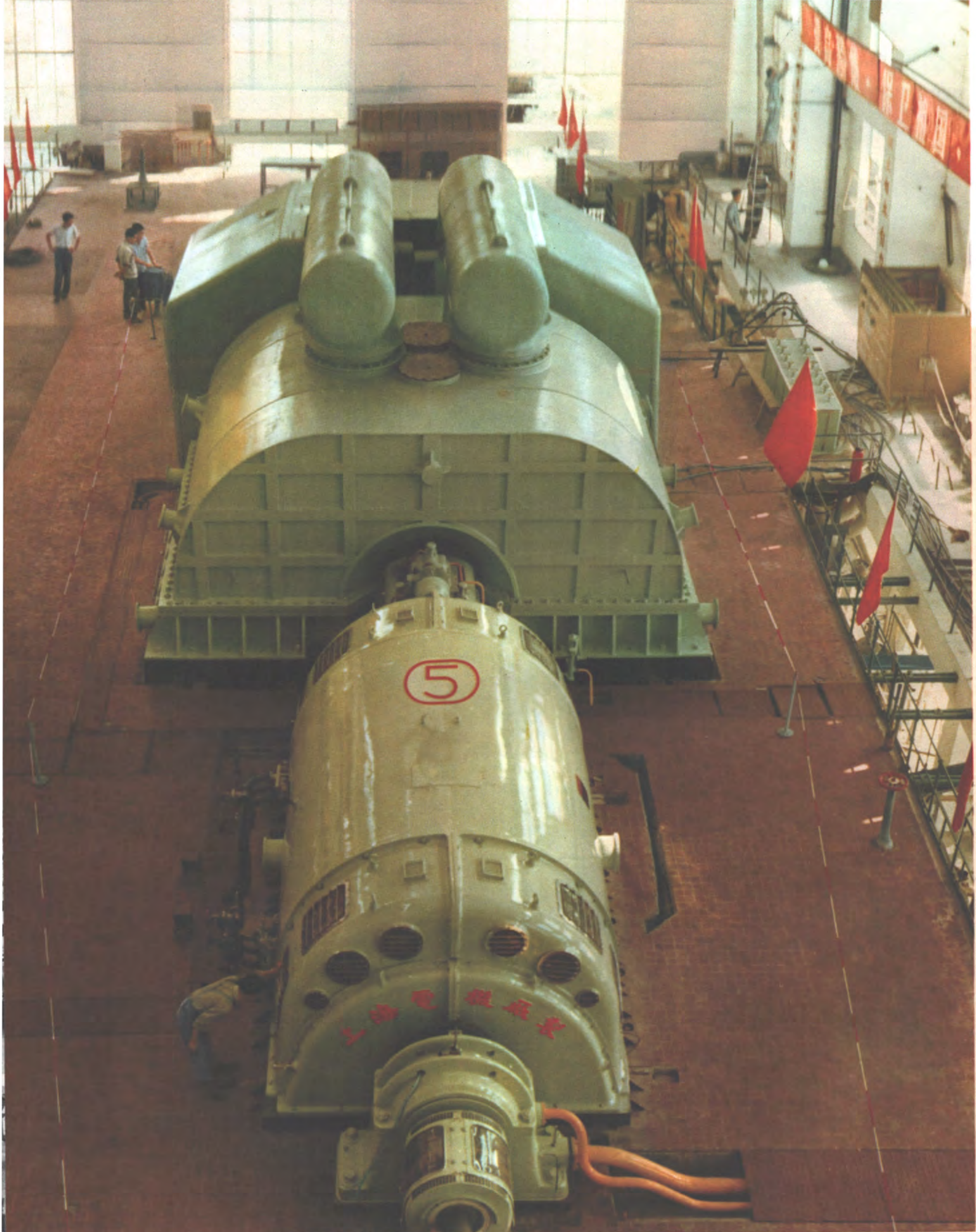
The 125,000-kw. steam turbo-generating set with a double internal water-cooling system, manufactured by the Chinese working class armed with Mao Tsetung Thought, is now in operation.
