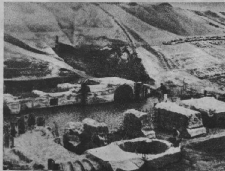
The lock at Huaiyin which was damaged by the Japanese and puppet forces during the War of Resistance to Japanese Aggression, is now under repair
