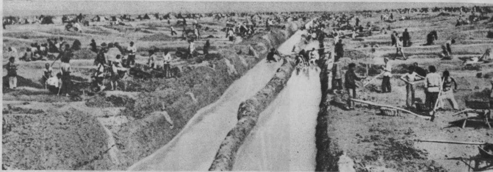
Nature's blunder was to give the Sui a winding course—a canal 30 kilometres long and 65 metres wide is being cut through a rocky area
